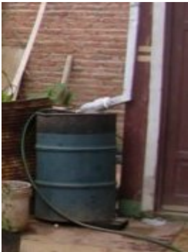
Figure 5-13. Rooftop rainwater collection equipment includes a drain from roof gutters, a turril , and a pipe that extends to a water tank underground.
