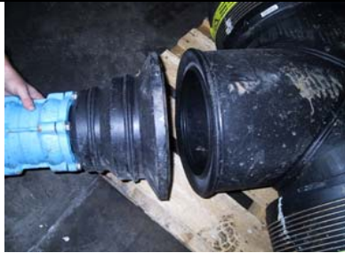
Split adjacent to butt weld
