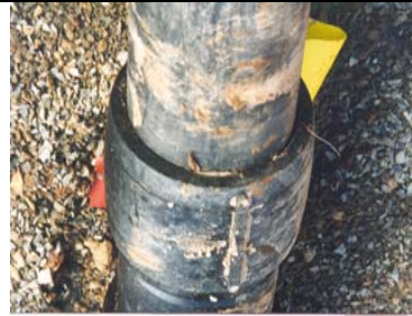
Leakage from electrofusion fitting
