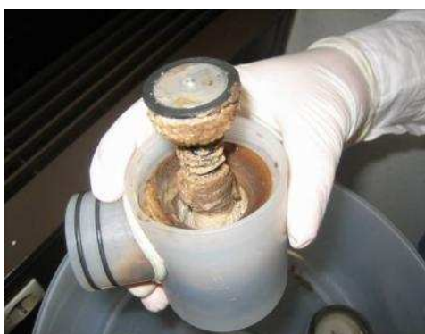
Fig. 9: Soft urine precipitations inside a urine valve of a Roediger urine-diversion toilet. This valve was disassembled and cleaned after clogging (source: L. Ulrich, December 2008). One valve costs EUR 118 and requires a bowden cable costing EUR 51(location of valve in Fig. 7).
