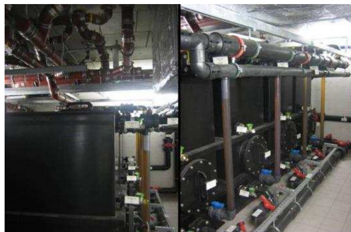
Fig. 5: Left: Plastic urine storage tanks in the basement of House 1 with connected urine pipework. Right: urine tanks with level indicating plastic pipes (source: L. Ulrich, April 2009).
