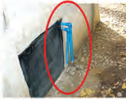
IMPROPER DISCHARGE OF GREYWATER & CLEANSING WATER
