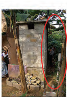
TOO CLOSE TO FENCE
