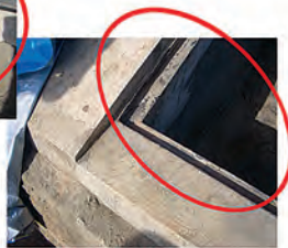
POOR DESIGN OF SLOPING COVER ALLOWING RAINWATER TO ENTER PROCESSING CHAMBERS
