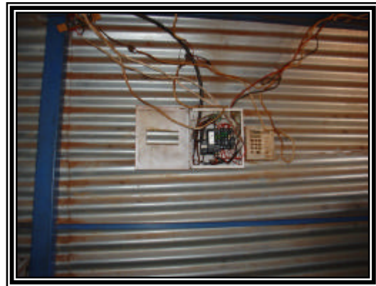
Even the church takes advantage of the illegal electricity connections
