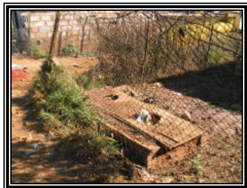
It has conclusively been proven that nitrate loaded effluent from pit latrines is directly responsible for widespread contamination of valuable groundwater resources.
