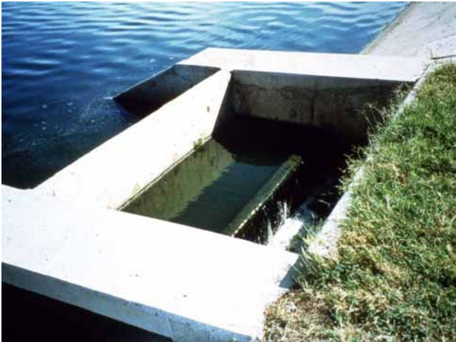
Figure 9. Pond outlet weir with integral scum guard.
