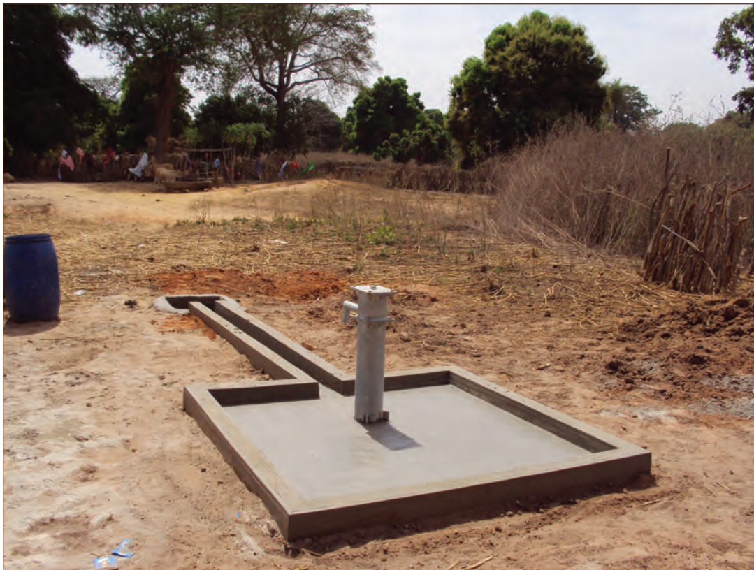
Concrete Apron and Hand Drilled Well
