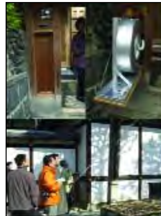
Fig. 27. Image of hydrant system for citizens (first fire-fighting phase)
