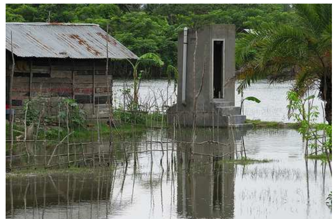
Figure 1: Urine Diversion Dehydration Toilets (UDDT) withstood the flood waters that resulted from a cyclone that struck southern Bangladesh in 2009 (source: A. Delepiere). More photos from this project: www.flickr.com/photos/gtzecosan/sets/72157626407064863/
