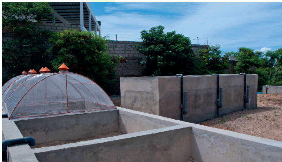
Figure 7.6 Pilot scale research facility at Cambérène treatment plant, Dakar, Senegal. Evaluating rates of dewatering with passive and active ventilation with greenhouses (photo: Linda Strande).
