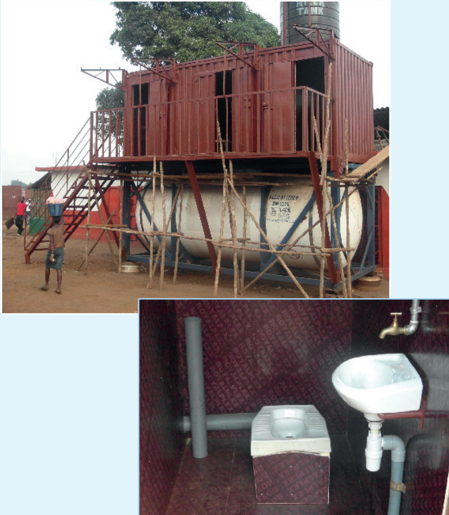
Figure 4.17 Large capacity modular and multi-functional transfer station (top), and sanitation facility (bottom) (photo: GOAL).
