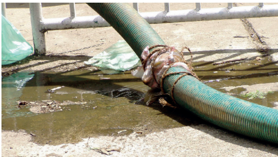
Figure 4.4 Hoses and fittings require frequent attention and repairs to keep them functioning properly. This picture illustrates inadequate maintenance, resulting in leaking of FS from the emptying hose (photo: David M. Robbins).
