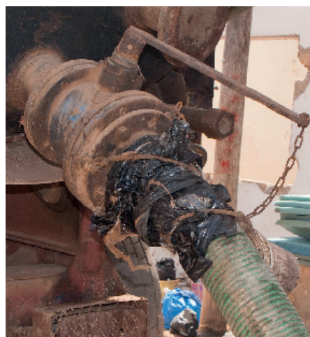
Figure 4.13 Example of an improperly maintained hose held together with plastic bags and twine (photo: David M. Robbins).
