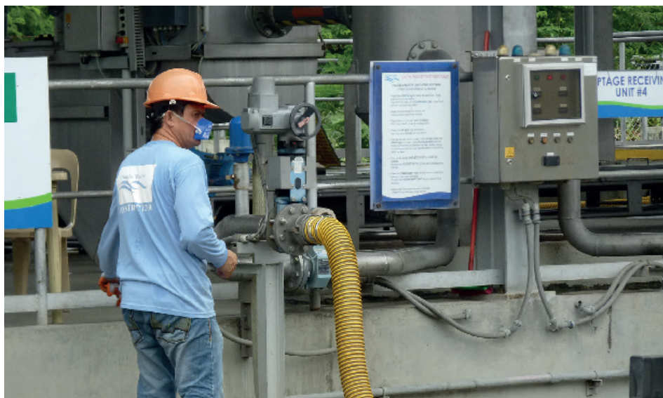
Figure 4.16 Automated faecal sludge receiving station at Manila Water's South Septage Treatment plant, Manila, Philippines (photo: WSUP, Sam Parker).
