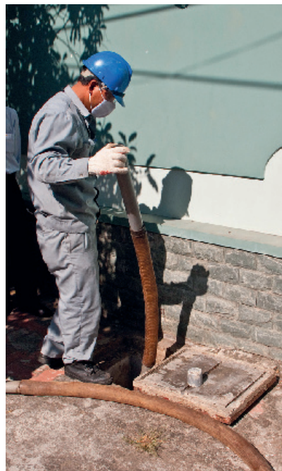
Figure 4.3 Example of a septic tank access port designed for ready access, Vung Tau Province, Vietnam (photo: Linda Strande).
