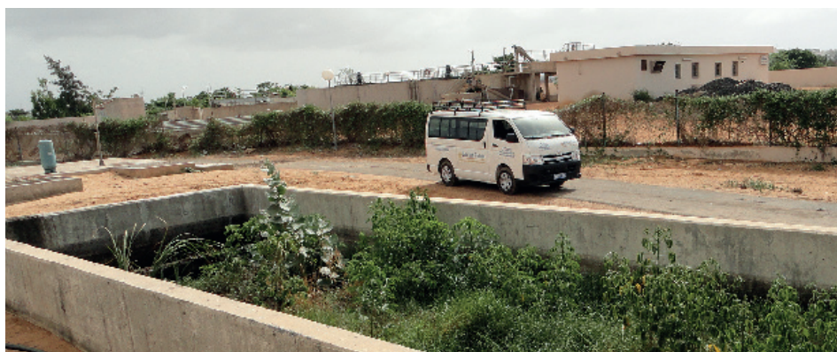
Figure 6.5 Example of inadequate operation and maintenance of a settling-thickening tank in West Africa. The scum was not removed during a long period, which allowed plants to grow on it. The volume of sludge and scum accumulated does not allow for proper operation of the tank, or for solids-liquid separation (photo: SANDEC).
