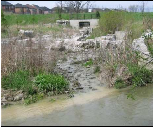
Outlet of a Retention Basin
