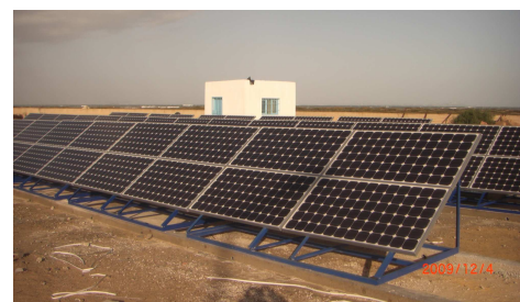
Fig 6 Photovoltaic Modules of the demonstration facility
