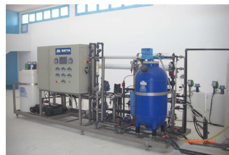
Fig 5 Reverse Osmosis Plant of the demonstration facility
