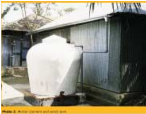
Ferrocement tank storage- Bangladesh
