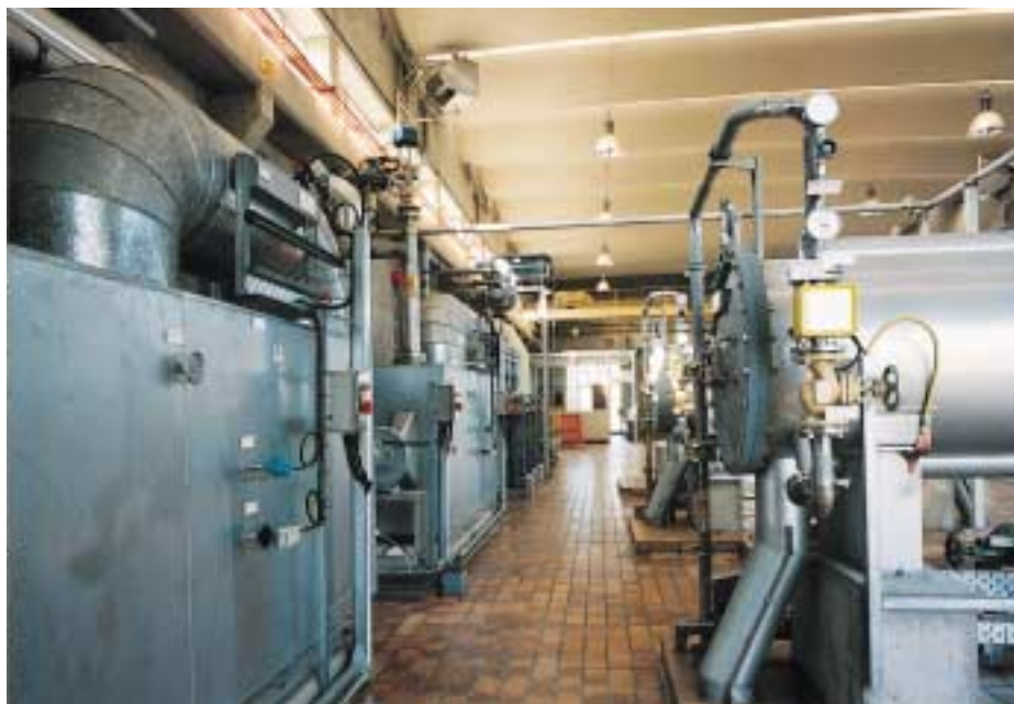
Figure 1: Loftsome Bridge WTW 2 x 9.5 kg ozone/h and vent ozone destructors
