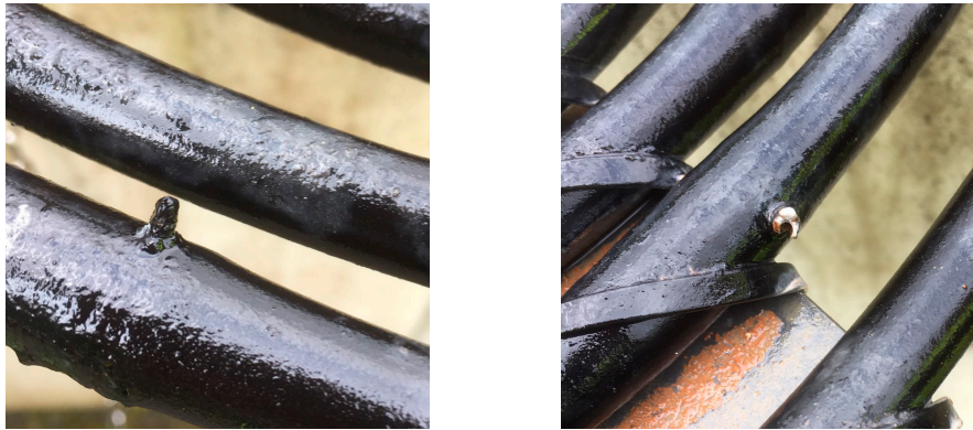
Figure 5. Blocked emitter orifices from an aerated wetland treating landfill leachate.
