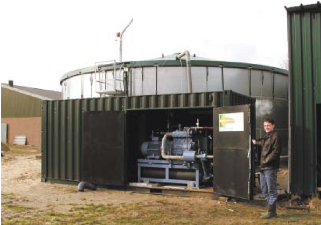
Figure 13. Biogas plant for manure digestion Praktijkcentrum Sterksel, The Netherlands. Photo by courtesy of www.energieprojecten.com .
