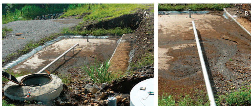
Figure 27. Sloughed sludge on the constructed wetland (CW) at Salazie, Réunion.
