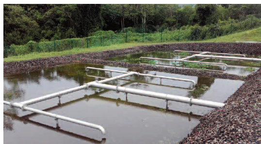
Figure 13. Recharge of the Taupinière facility filters during tropical storm Matthew. It is the facility's second-line filters that are not yet in service, and so not replanted, as the system is under-loaded.
