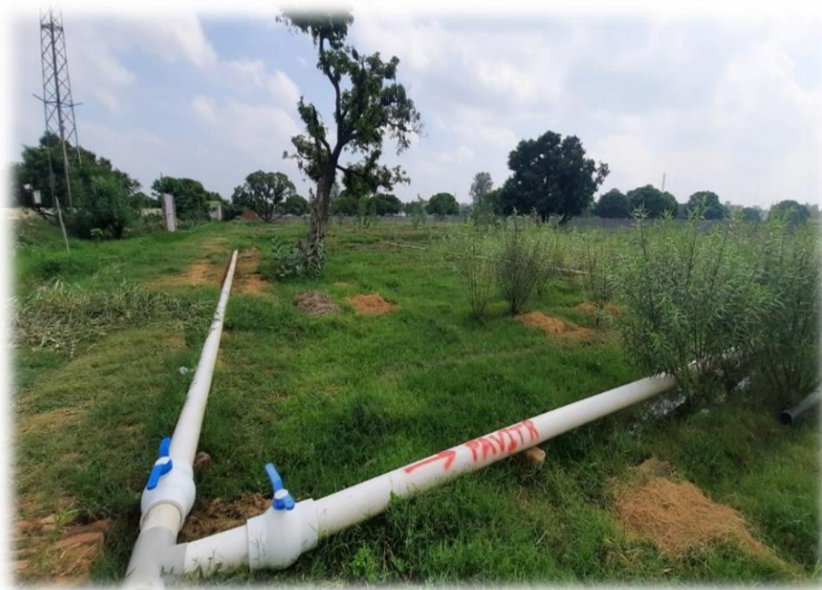
Wastewater Transport System
