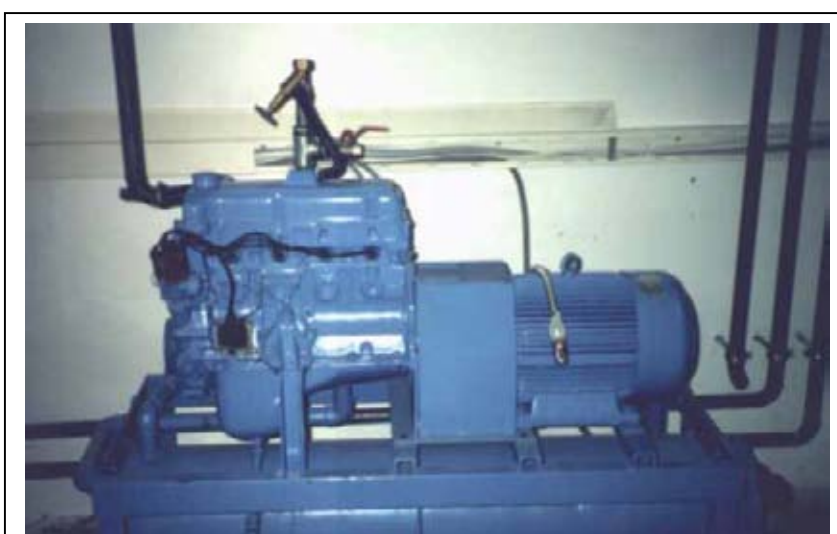
Figure 47: Co-generation unit (electricity and heat utilisation)
