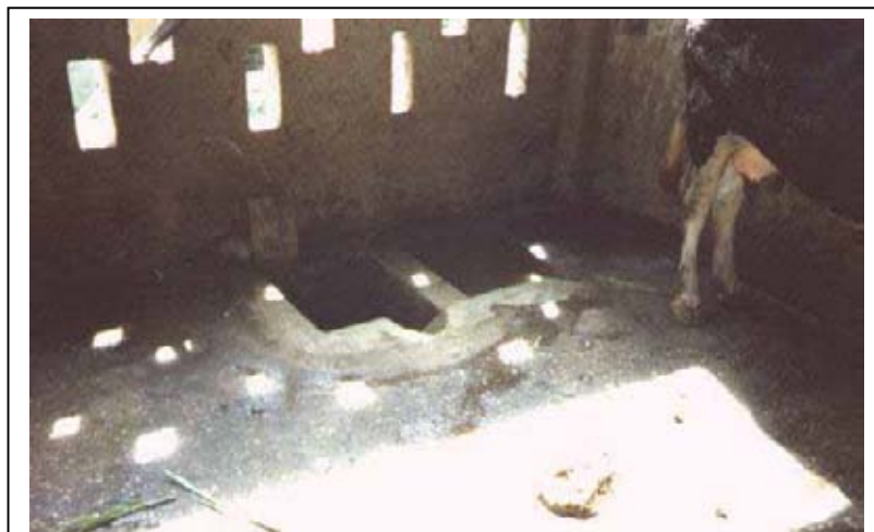
Figure 23: Cowshed, directly connected to the plant: A urine chamber to the right collects the liquid which can be used to wash the dung into the digester.
