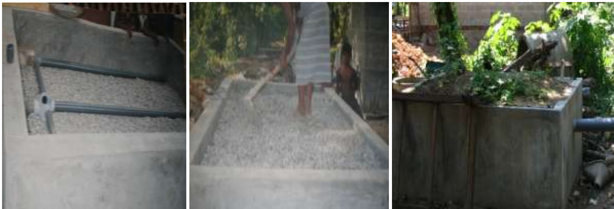
Vertical filter under construction (left and middle), planted filter in operation (right) – Thotagamuwa, Sri Lanka
