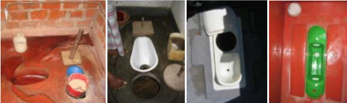
Dry, urine diversion toilets in Sri Lanka, with pipe for urine and wash water infiltration
