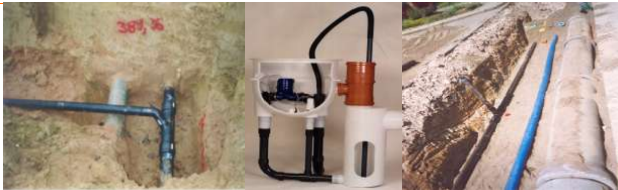
HDPE Vacuum Pipe with individual connection (left), collection chamber (centre), wastewater collection, water supply and storm water drainage pipes in one trench (right)
