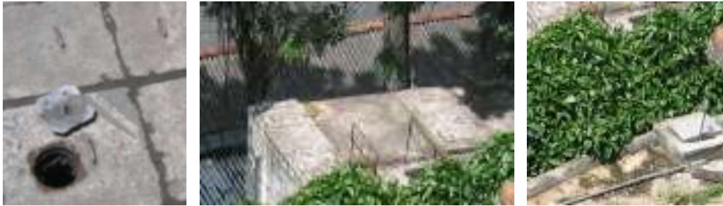
inspection opening, baffled anaerobic filter, constructed wetland with effluent reuse (irrigation & car washing), Kandy, Sri Lanka
