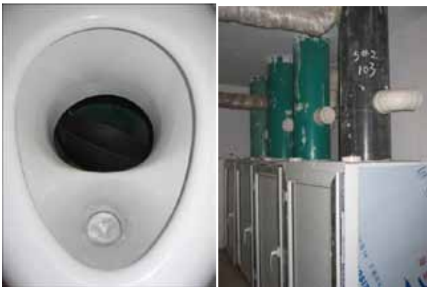
Figure 18. Left : Ceramic urine diverting dry toilet equipped with faeces turning bowl and odour trap for urine. Right : Downpipes coming from each floor leading into separate bins with housing (Erdos Eco-Town, Dong Sheng, China, photos: W. Berger, 2009)
