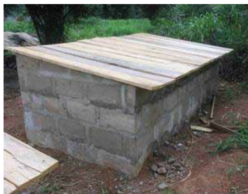
Figure 2. Brick chamber for faeces composting equipped with vent pipes on the back side and sheltered (photo: W. Berger, 2009 at German Research project at Valley View University, Ghana)
