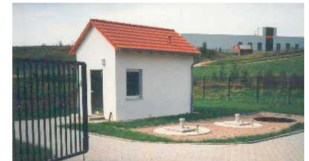
Figure 6: Vacuum station with buried vessel
