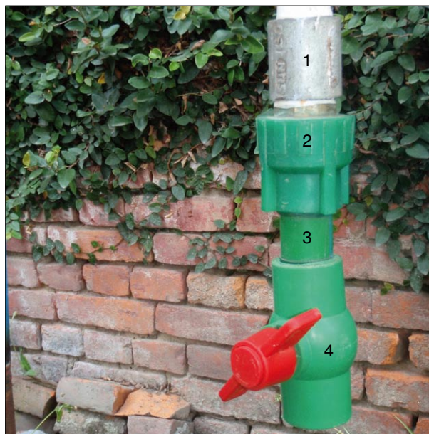
Figure 14: Detail view on the lower reactor outlet from the sheet metal tank to the PP ball valve
