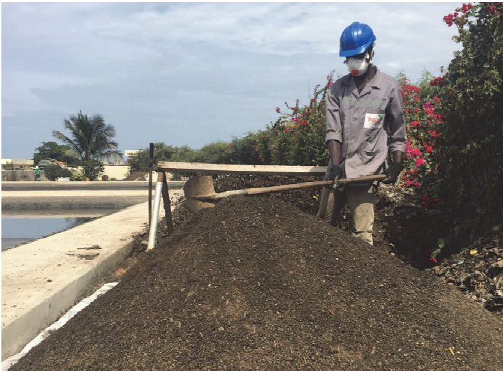
Figure 2.3.6 Faecal sludge treatment plant in Dakar, Senegal.
