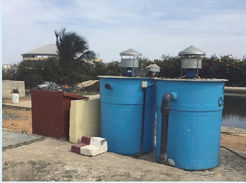
Figure 3.7.1 The flocculation unit at a faecal sludge treatment plant in Dakar, Senegal. Operated by DELVIC Sanitation Initiatives.
