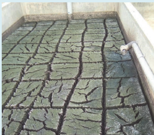
Figure 3.3.3 Pathways created in the sludge cake to increase exposure to heat and sunlight.
