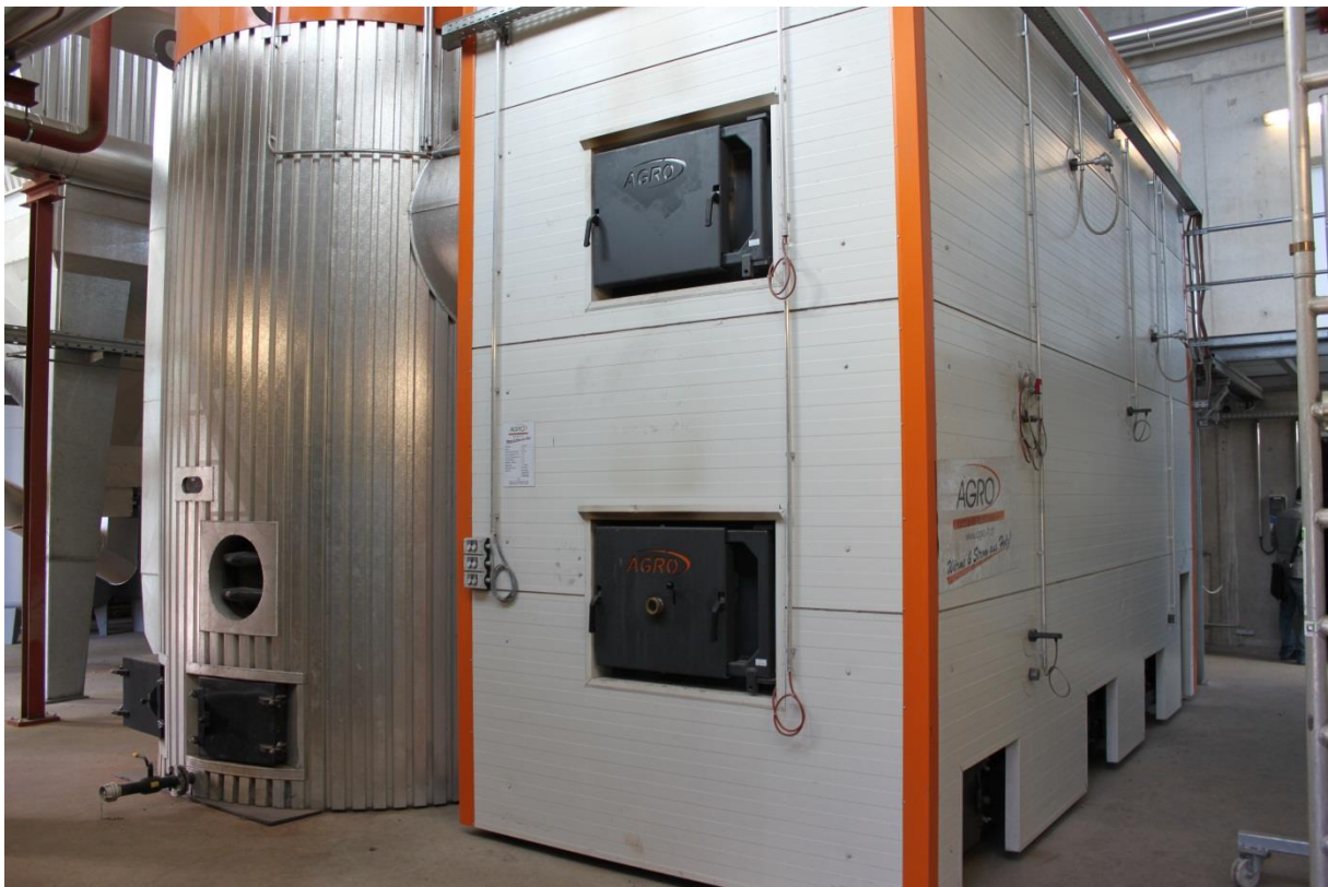
Figure 62: Medium sized woodchip heating system (3,000 kW heat capacity) with the boiler (right) and the buffer tank (left) of the Biomassehof Achenal in Germany (Source: Rutz D.)
