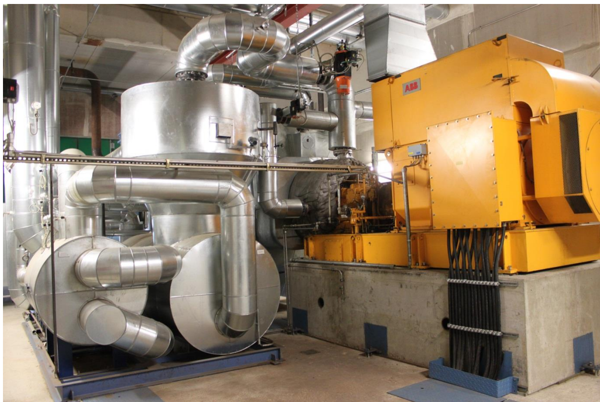
Figure 63: ORC system (1,520 kWel) of the Grünfüttertrocknungsgenossenschaft Kirchdorf a.H. eG in Germany (Source: Rutz D.)
