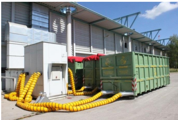
Figure 47: Container and air heating pipes for woodchips drying at a biogas plant in Munich, Germany (Source: Rutz D.).
