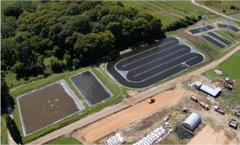
Figure 2 Photograph of a covered anaerobic HRAP system in the Waikato, New Zealand.
