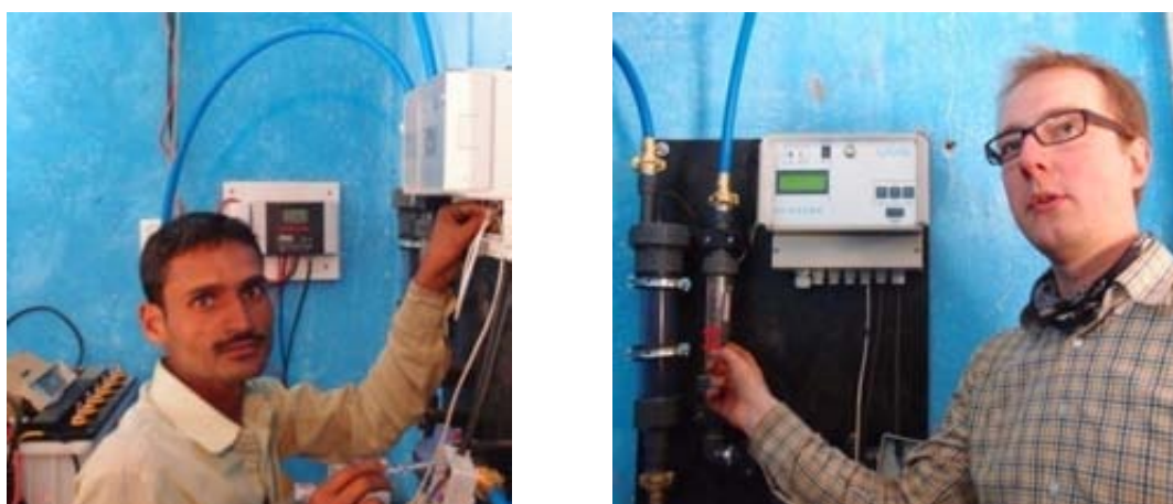
Figure 23: Installation and Explanation of AO Disinfection System.
