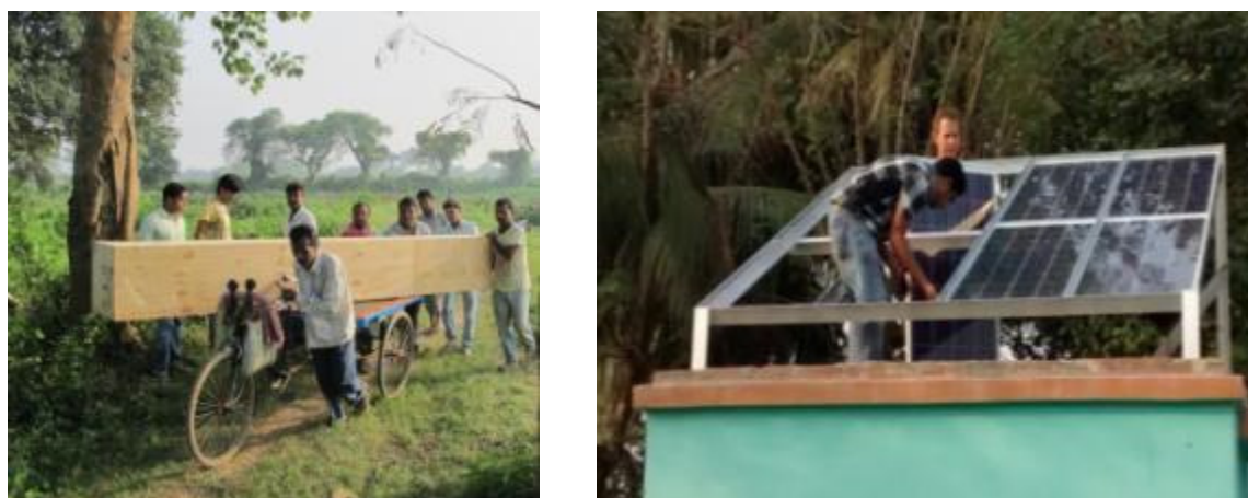
Figure 17: Transport of PV substructure and installation of PV System at KALYANI site.
