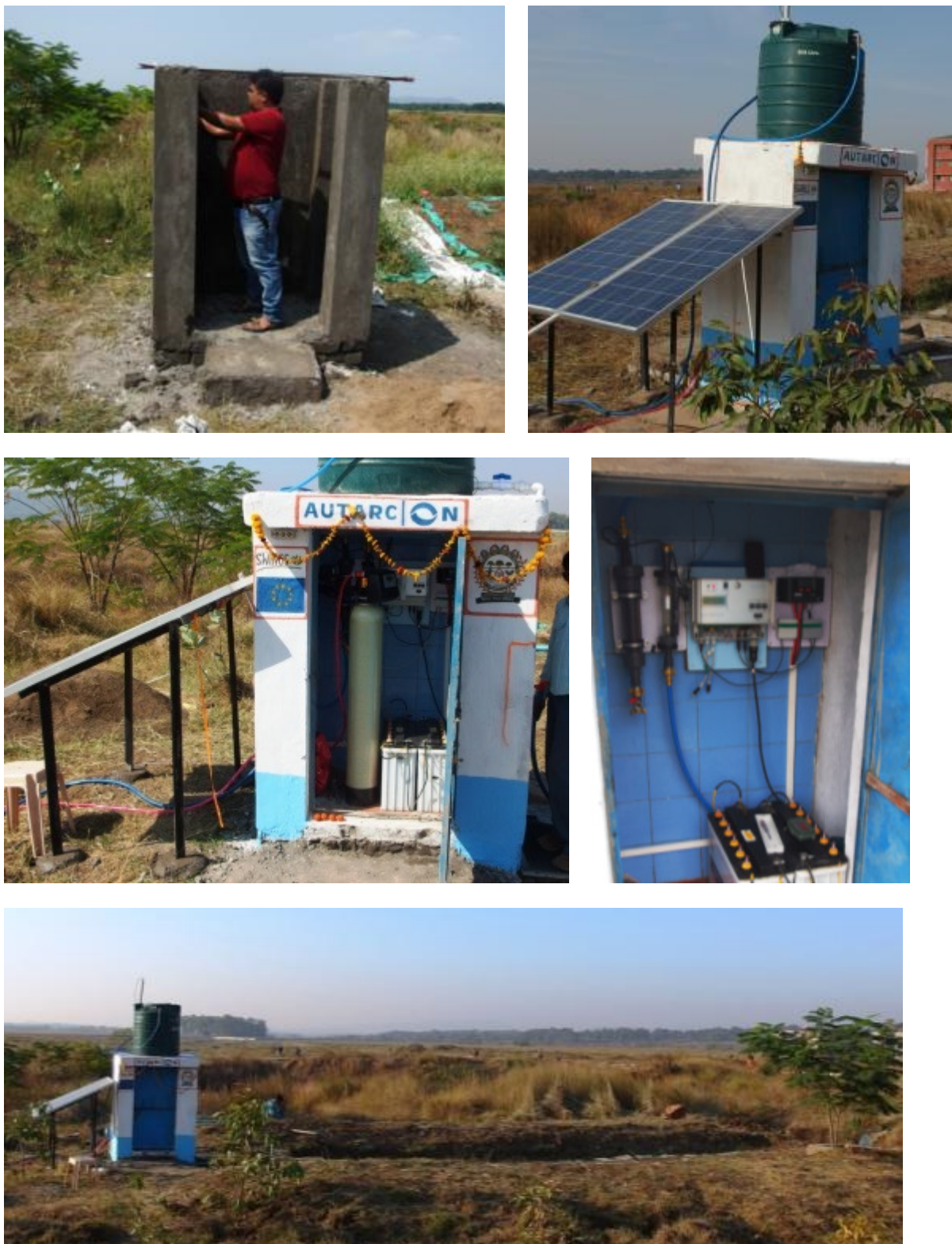
Figure 28: Construction of building for water tank and solar panels and installation of disinfection unit at Amarkantak (IGNTU Campus site).
