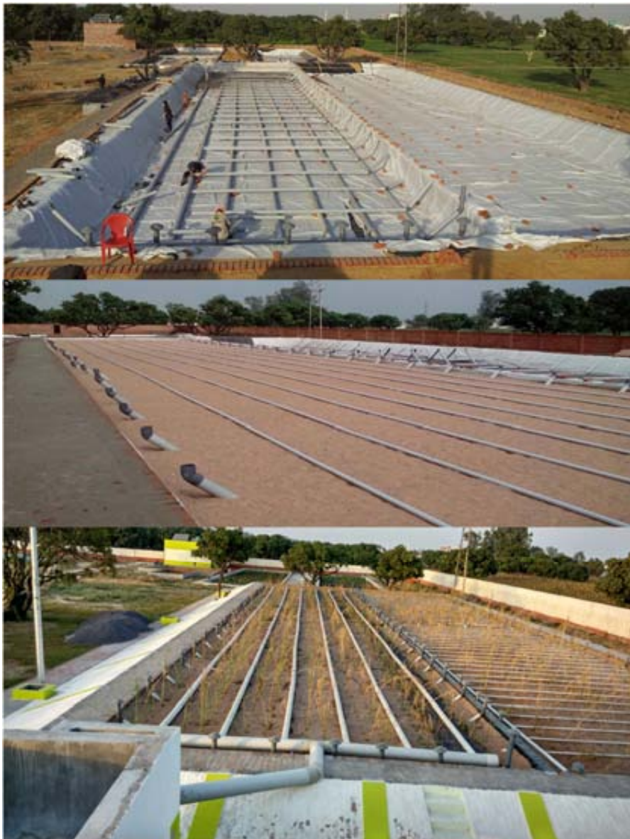
Figure 4: Implementation phases of vertical constructed wetlands in large AMU pilot plant.
