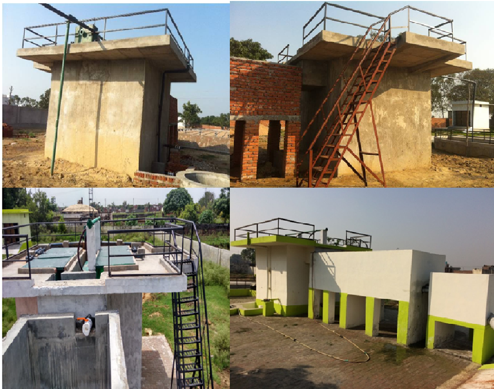
Figure 2: Implementation steps of UASB reactor at large AMU pilot plant.
