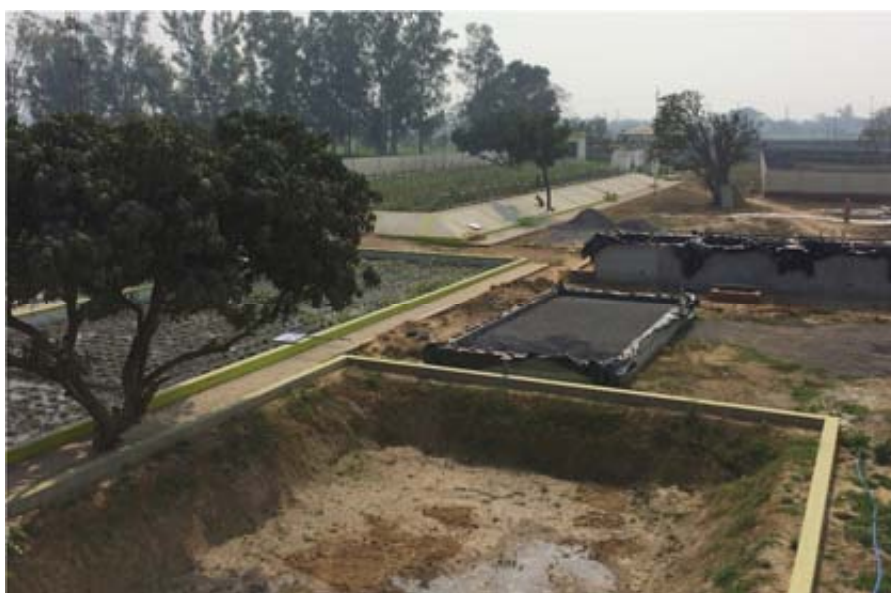
Figure 11: View of the whole FS under construction, including VF bed, HF bed and maturation pond. To the left the large AMU pilot plant in operation can be also observed.
