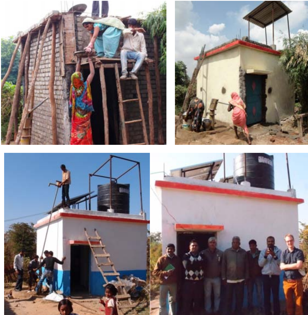
Figure 21: Construction of the water tower structure at Lalpur disinfection pilot plant (IGNTU site).
