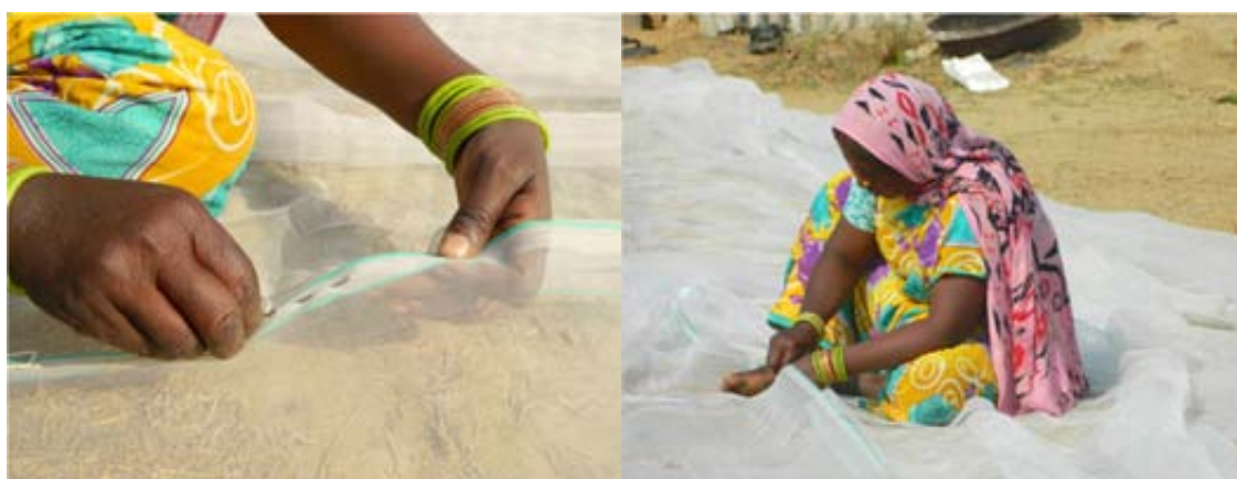
Figure 9: Sewing the geotextile for the VF beds of the FS pilot plant.
