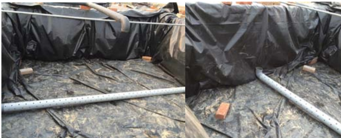
Figure 7: View of the installation of the distribution pipes (left) and the draining pipes (right).
