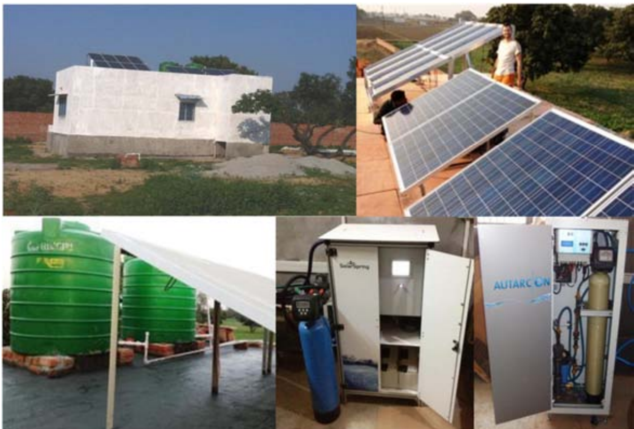
Figure 6: Laboratory building, solar PV panels, water tanks and UV and AO disinfection systems implemented at large AMU pilot plant.
