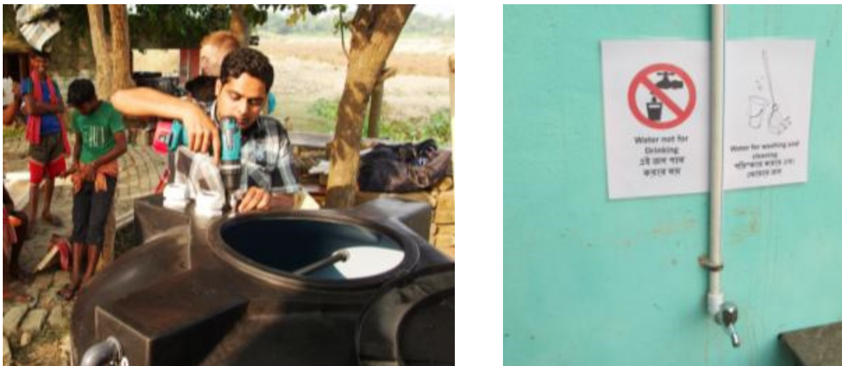
Figure 18: Water tank installation and sampling taps.
