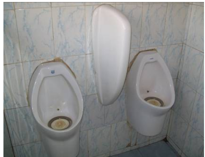
Figure 4. Urinals with sealant liquid based odour traps (Photo:R.Sakthivel)
