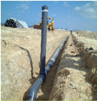
Vacuum sewer line with inspection point
