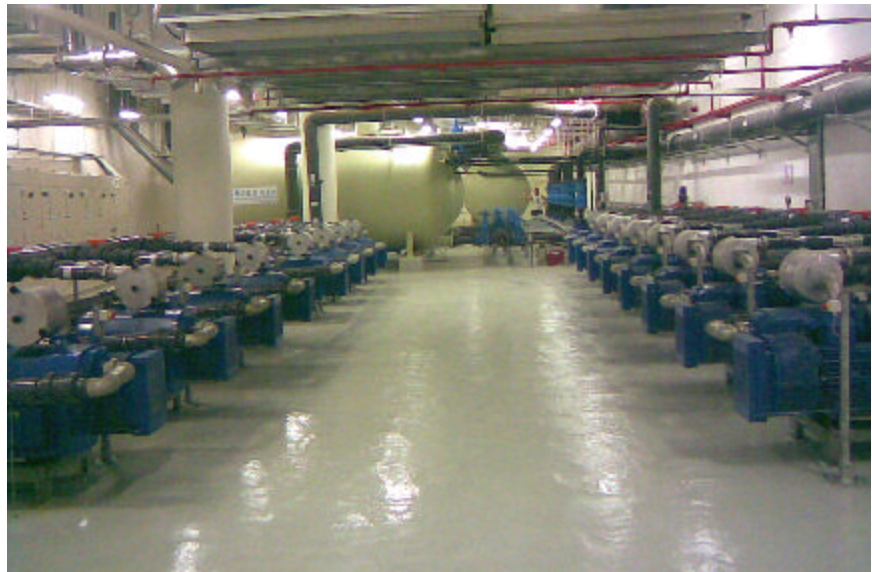
Vacuum Station with Vacuum Tanks
