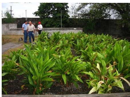
The DEWATS horizontal gravel filter can be aesthetically incorporated in the local surroundings. Dumaguete Public Market
