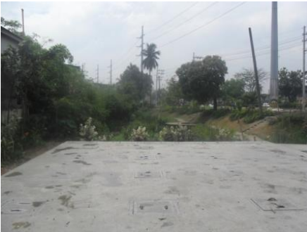
The surface of the decentralized underground DEWATS system can be used as parking space. Pabahay sa Riles Paco, Manila
