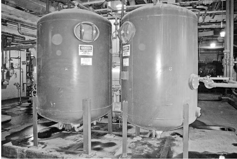
Figure 10-11 Example of full-scale anion and cation exchange columns.
