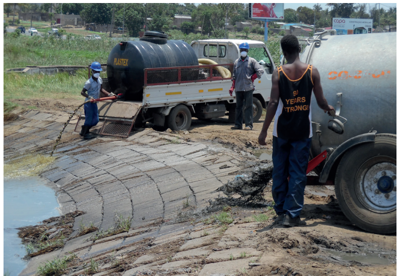
Image: FSM business disposes of waste at the centralised treatment plant, Maputo.
