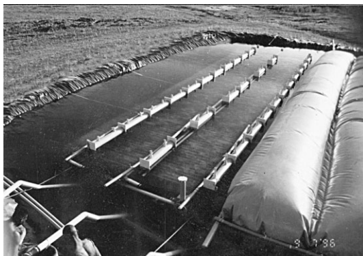
500 m 3 UASB-Reactor for Cane Sugar Wasterwater Treatment, Jamaica
