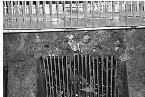
Manually cleaned screens/bar rack St. George's University Grenada (Daniel and Daniel Engineering Inc.)
