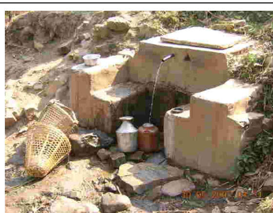
Outlet pipe from an 'open system' protected spring in a hill district in Nepal
