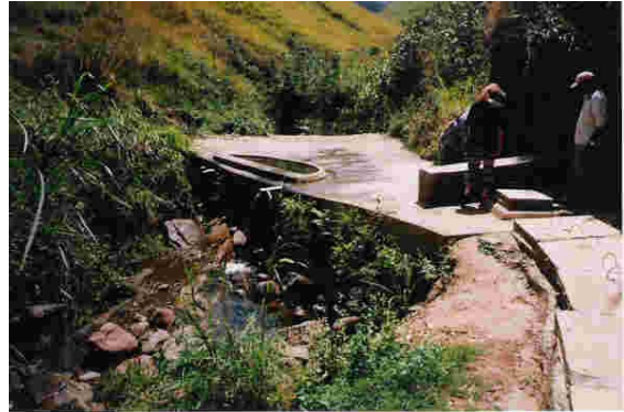
Spring box with roughing filter on the outlet (to the right) prior to the water entering the pipeline
