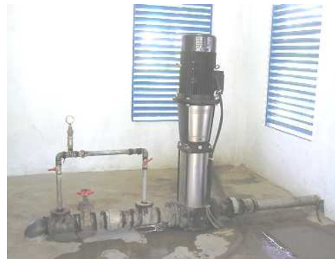
The electric pump
