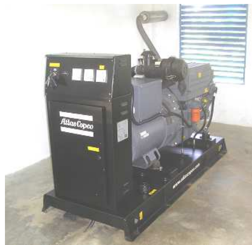
The diesel generator
