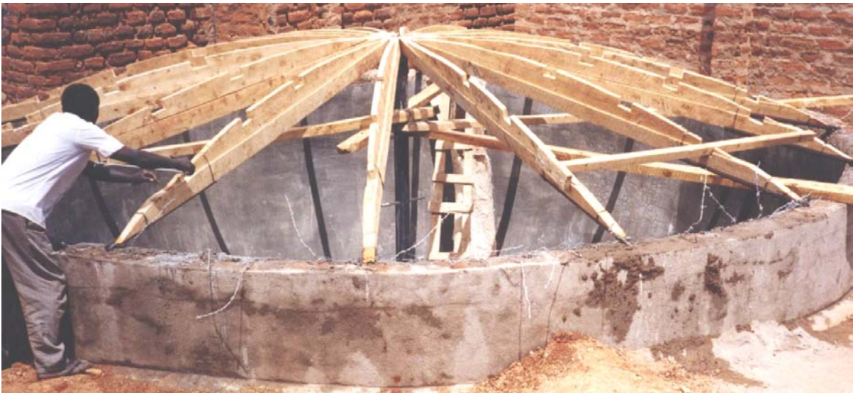
Reusable formwork being assembled for a dome on a hemispherical tank built of ferro-cement with a storage volume of 90,000 litres during a training course in Namibia.
