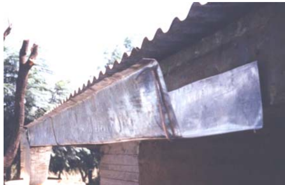
Square gutter fixed without splash-guard.
