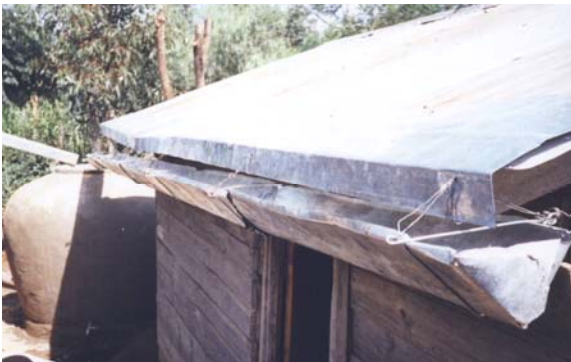
V-shaped gutter suspended from a splash-guard.
