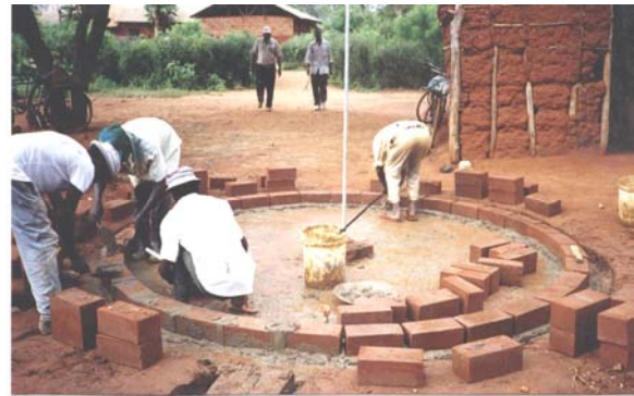
A water tank being built of compressed soil blocks during a training course in Kenya.
