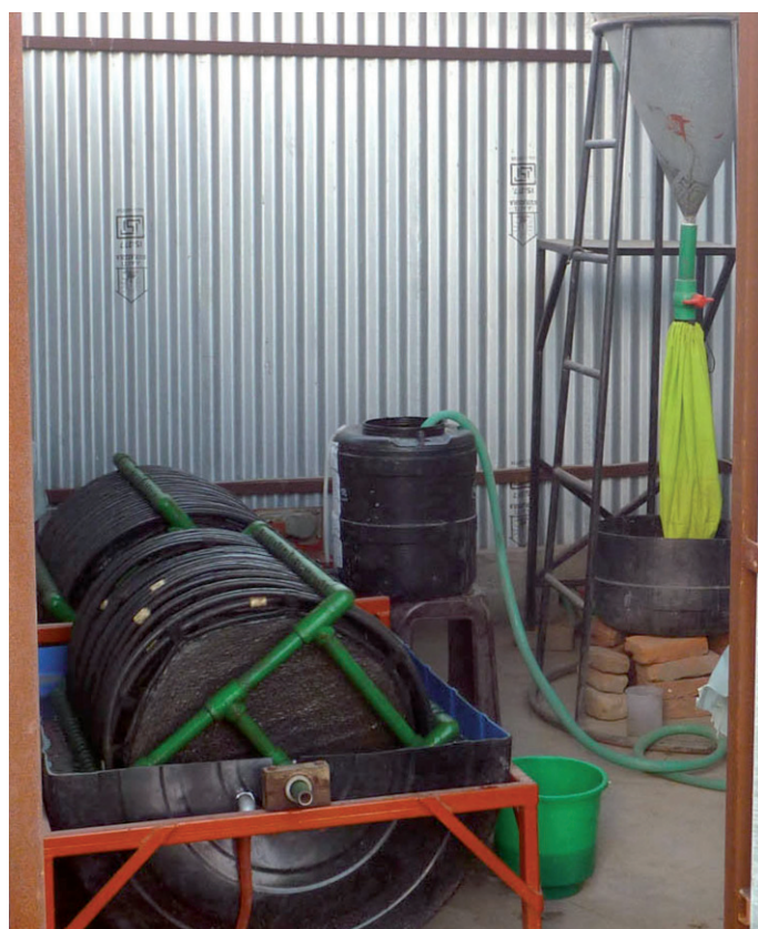
Figure 1: The rotating biological contactor (foreground left) and the struvite precipitation reactor (background right).
