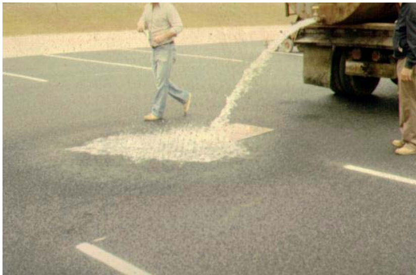
Porous Pavement Infiltration. Testing new pavement installation. Note: steady flow passes through pavement and into stone storage below with minimal spread.
