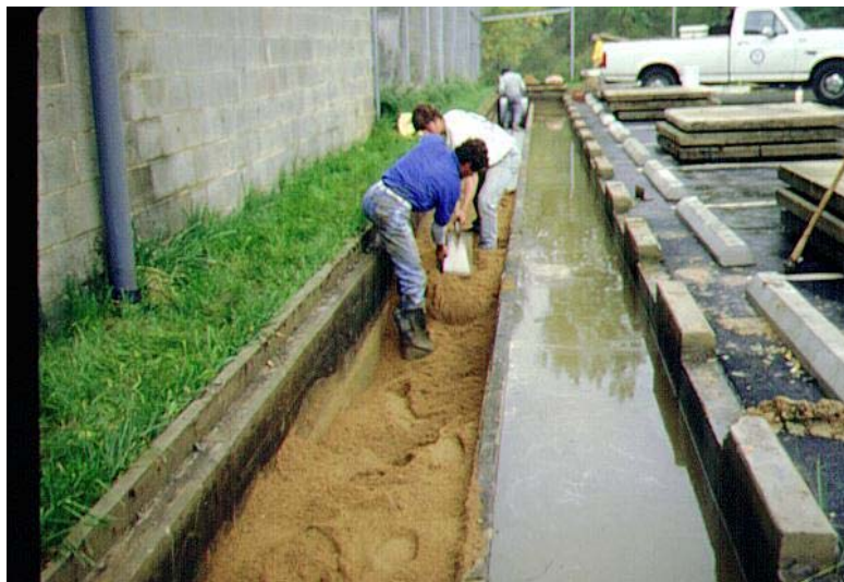
Sand Filter under construction. Note curb cuts for inflow to wet chamber with weir overflow into sand chamber.
