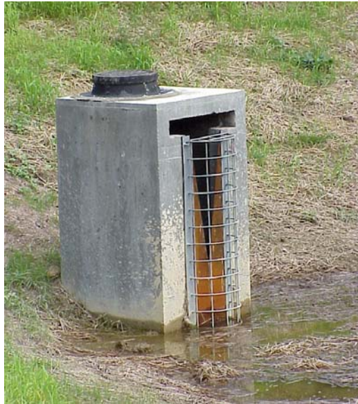
Principal Spillway multi-stage riser – “V” shaped weir protected by trash rack.
