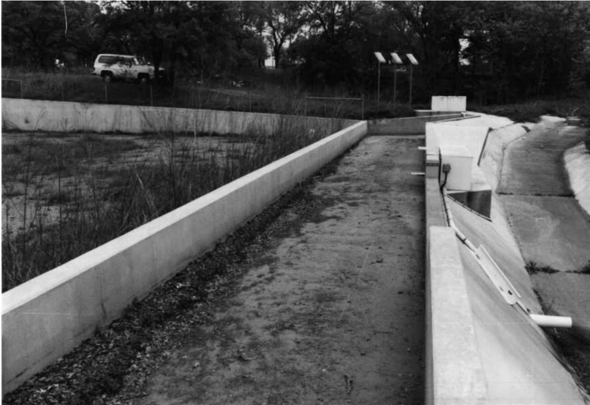
FIGURE 3.12C - 2 Sedimentation Basin of Jolleyville Partial Sedimentation System
