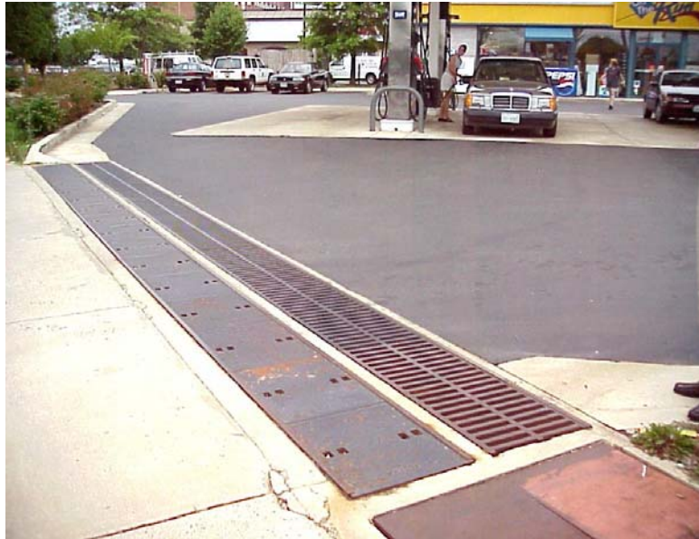
Sand Filter at entrance to service station.
