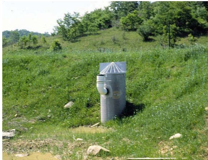
Principal Spillway multi-stage riser configured for temporary sediment basin function. Note anti-vortex plate and inclined trash rack to prevent clogging.
