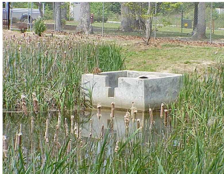
Enhanced Extended Detention Basin – Shallow Marsh. Note multi-stage weir principal spillway and deep water pool (18” – 48” depth).
