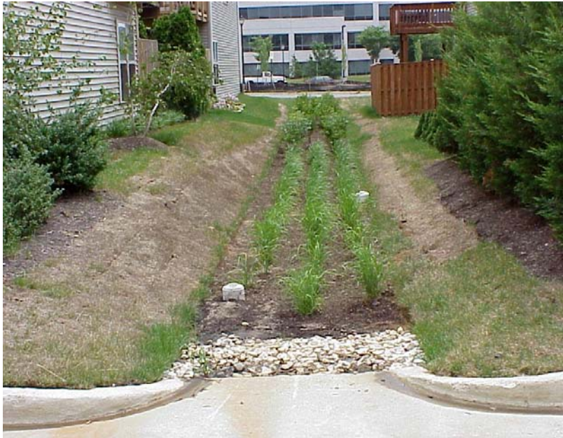
Bioretention Filter in ultra-urban setting. Note curb cut, gravel energy dissipater, and clean out/observation wells.
