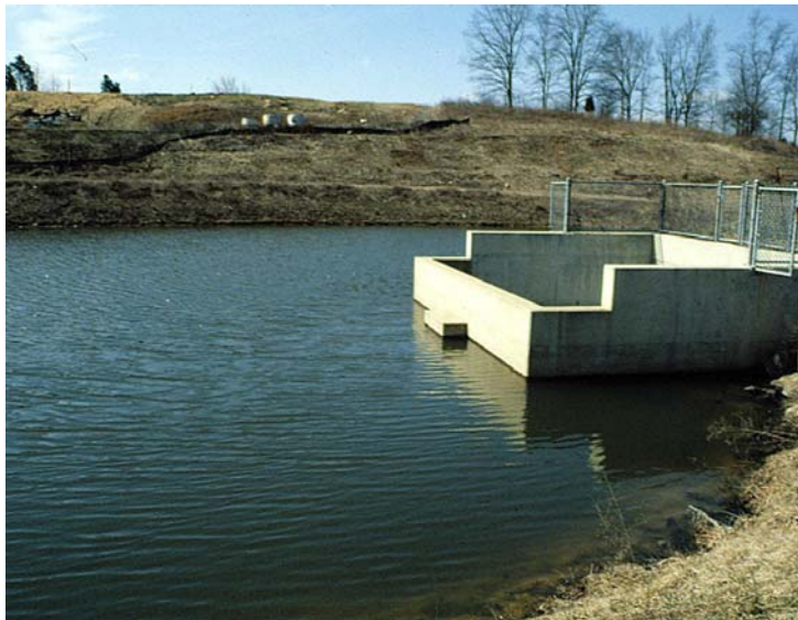
Principal Spillway multi-stage weir. Note low flow/extended detention orifice protected by “hood” draws water from approximately 18” below pool surface.
