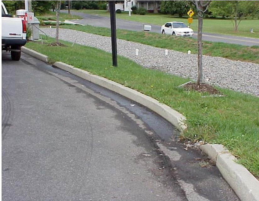
Surface Infiltration Trench. Note grass strip pre-treatment holds heavier particulate pollutants within paved area.
