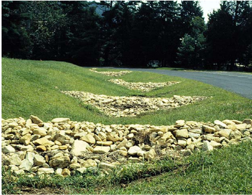
Grass Swale with Check Dams. Note significant channel storage capacity created by check dams. Notched center allows safe overflow without scour around sides.
