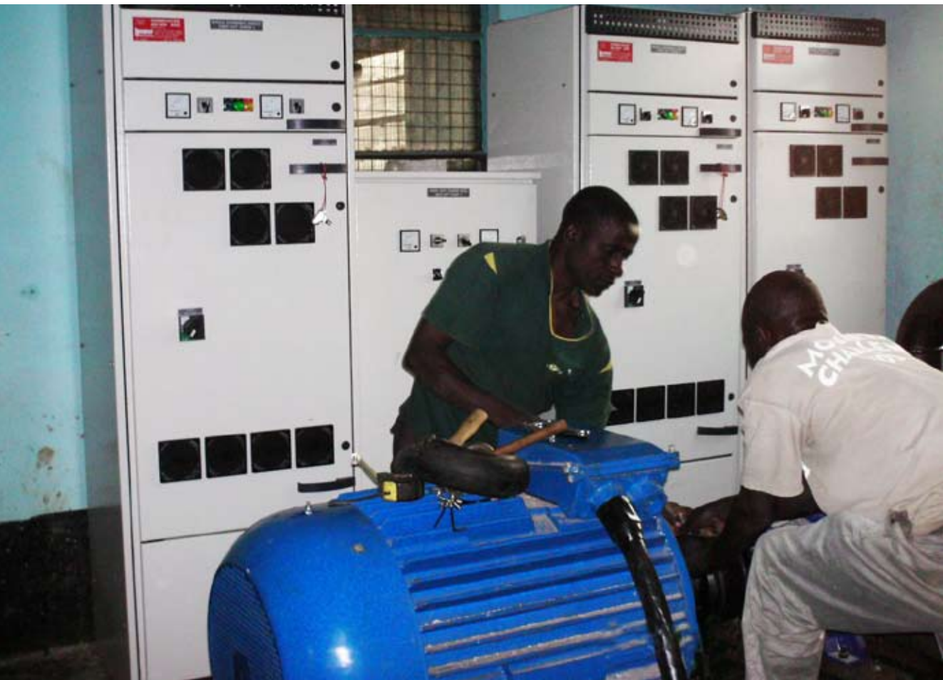
Routine maintenance in the water pump house. Photo © UN-Habitat
