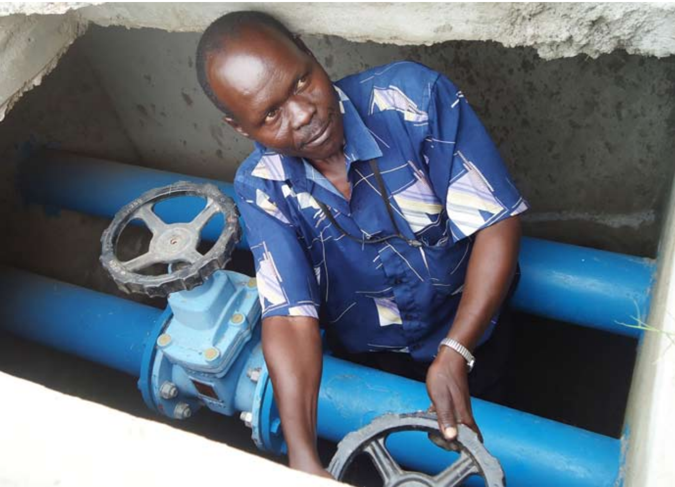
Checking the pump performance. Photo © UN-Habitat
