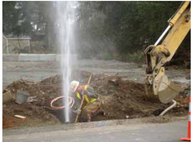
Chris Webster, a Tacoma Water utility worker, repairs a leaking distribution main. Tacoma Public Utilities Photo
