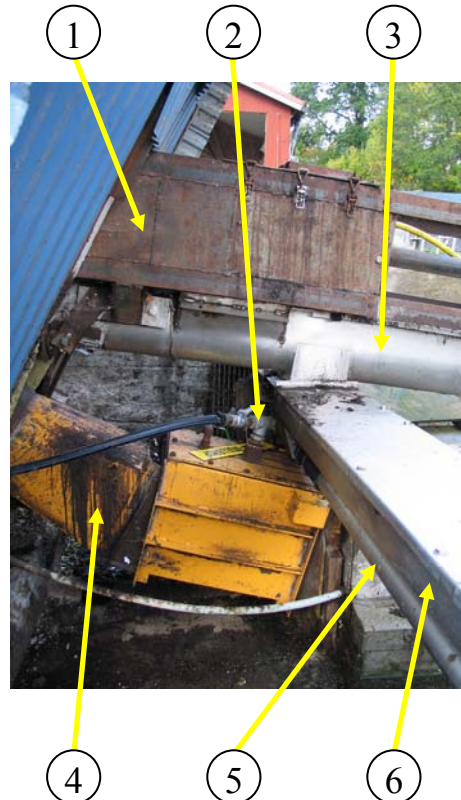
Figure 12. Filling and discharging the hydrolysis reactor. 1 frame of the drawer, 2 recycling of liquid fraction for lubrication of the feeder channel, 3 transport screw, 4 feeder channel, 5 drain pipe for liquid fraction, 6 extruder screw
