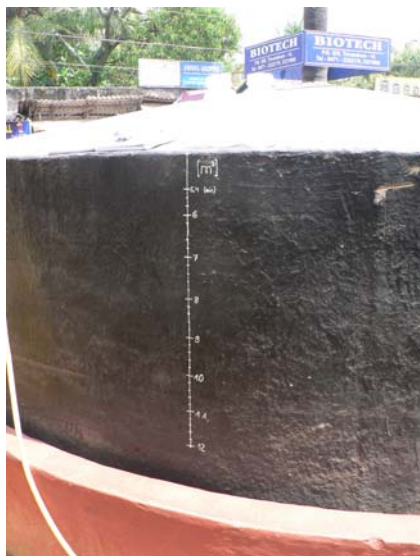
Figure 8: Scale for the gas content of the gasholder drum (Picture: Florian Heeb)
