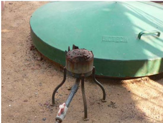
Figure 10: Excess biogas is burnt at the Sreekaryiam market level plant (Picture: Florian Heeb).
