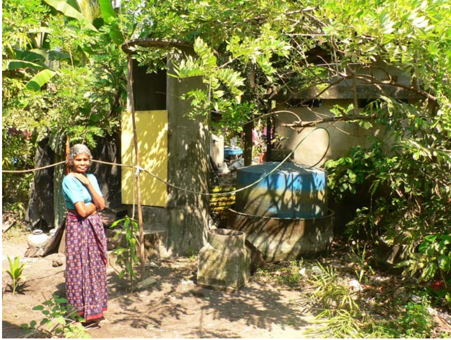
Figure 21: Toilet linked BIOTECH biogas plant on the island of Kumbalangi.
