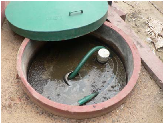
Figure 15: Effluent tank at the Sreekaryiam market level plant (Picture: Florian Heeb).
