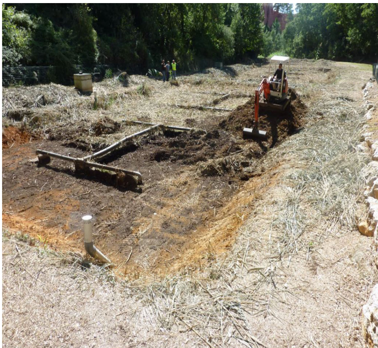
Figure 5.8 Sludge removal from the first stage French VF wetland in Roussillon, France after 13 years of operation (Troesch and Esser, 2012).
