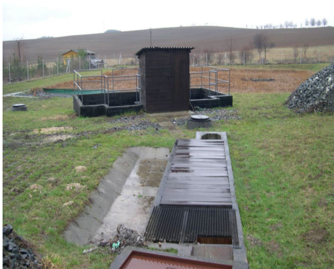
Figure 3.5 Ondřejov HF wetland: sand trap (front), Imhof tank and vegetated HF bed (back). Photo courtesy of Jan Vymazal.
