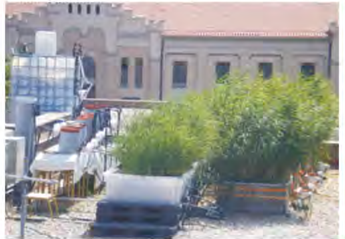
Fig. 2.3: Prototype of an integrated black water system UASB followed by a hybrid wetland in Barcelona, Spain. Source: UPC 2011
