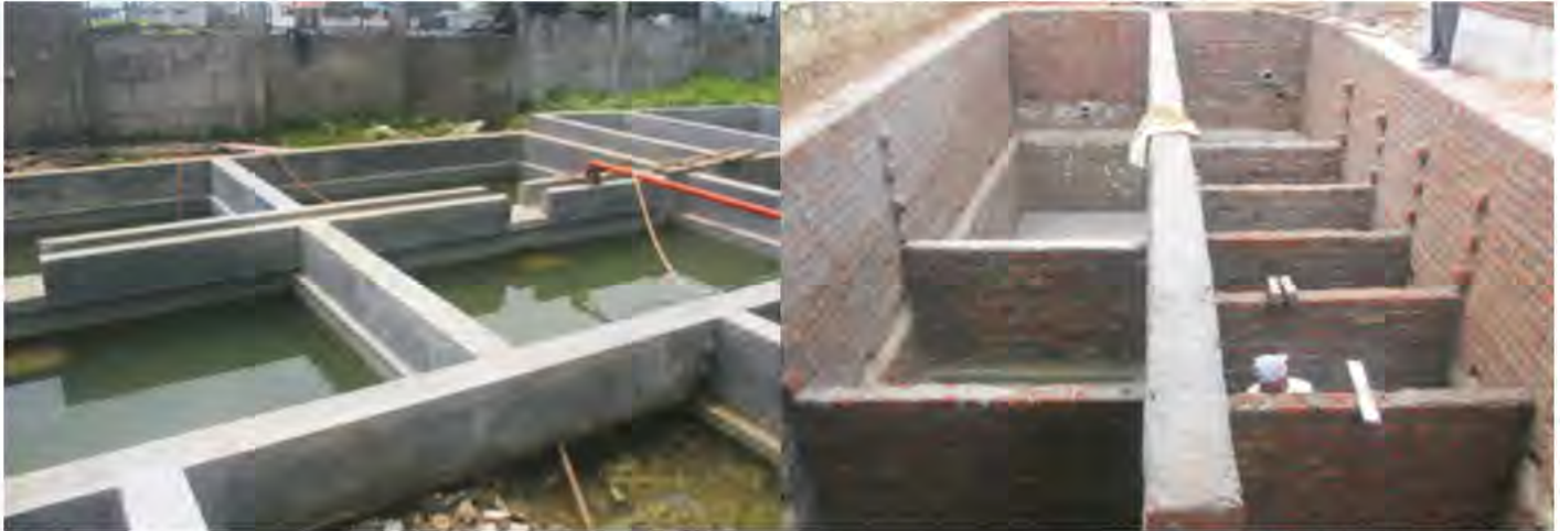
Photos by Barreto Dillon 2013 and 2010
