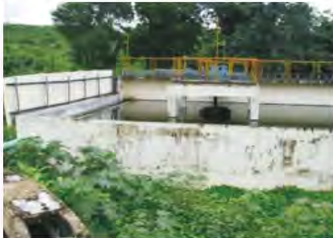
Fig. 2.1: Collapsed activated sludge wastewater treatment plant in Pandharpur, Maharashtra. Source: Barreto Dillon 2010
